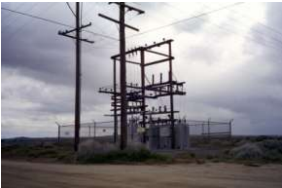
SCE North Muroc Sub-Station
